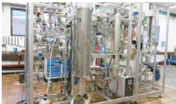
Main module of the new RWE pilot plant, status as of February 2023
